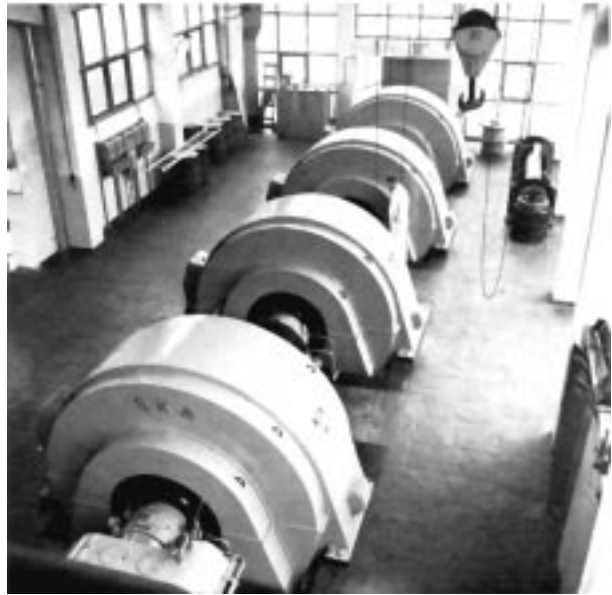
Fig. 2 Former main drive system
