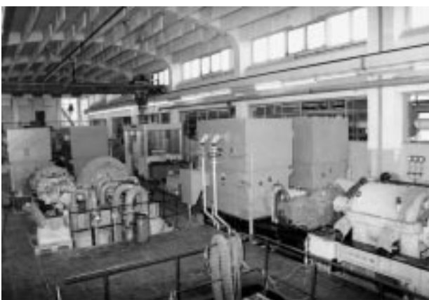
Fig. 16 Two 40-bar aircompressors driven by 2 DOL motors
