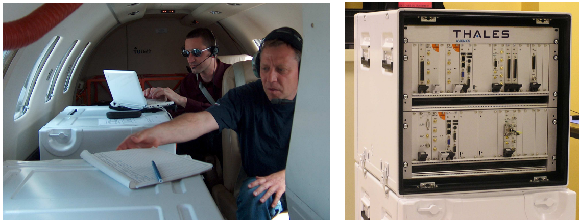
Figure 3 Left: Impression of cabin layout with the two white-coloured avionics boxes attached to the seat tracks. Right: One of the boxes opened in the workshop.
