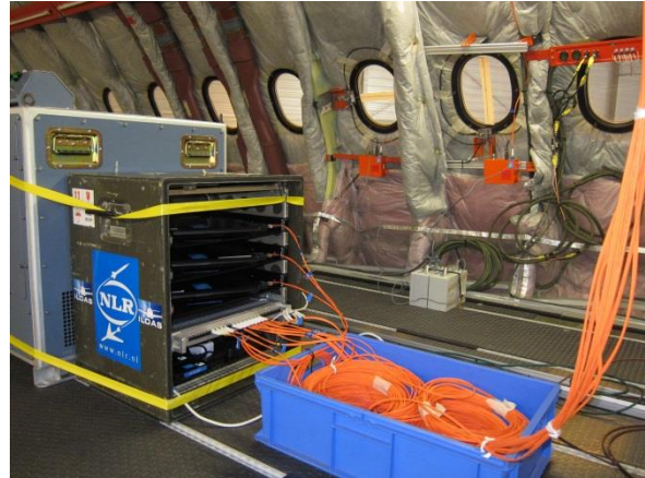
Figure 8 – Installation of the DADS equipment cabinet, and two window sensor installations (horizontal and vertical) in the background
