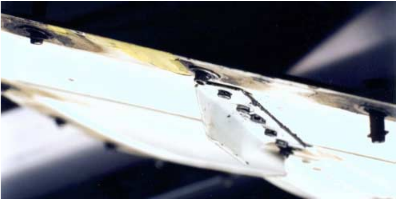
Fig. 3 Lower side of access panel 2408 with a stiffener repair
