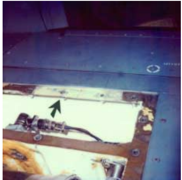
Arrow indicates location of cracks
